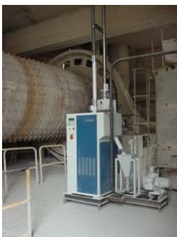
Air Tube Plant Station 发送站风动送样管道
